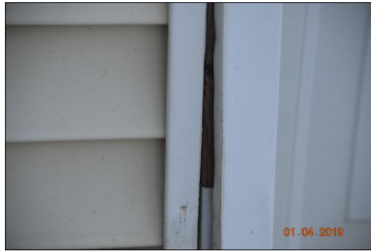
Loose/ damaged trim by garage door
