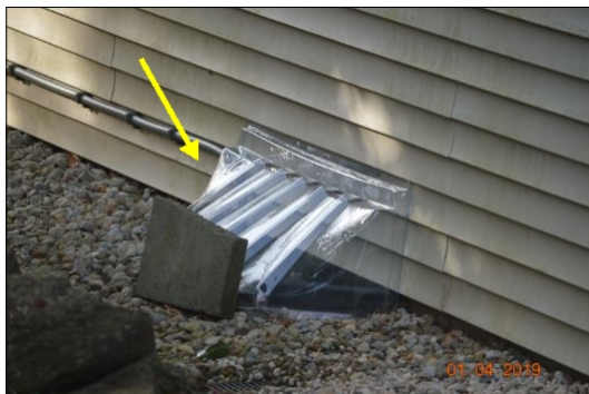
Loose window well cover
