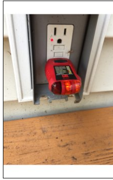
Non working gfi at rear of house.
