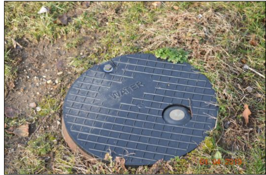
Water meter located in front lawn
