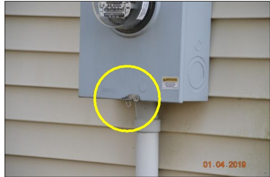
Missing power company service tag
