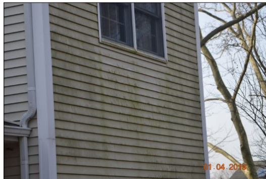
Maintenance needed - power washing
