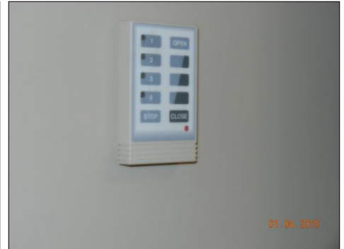
Skylight controls - 1 upstairs, 1 downstairs
