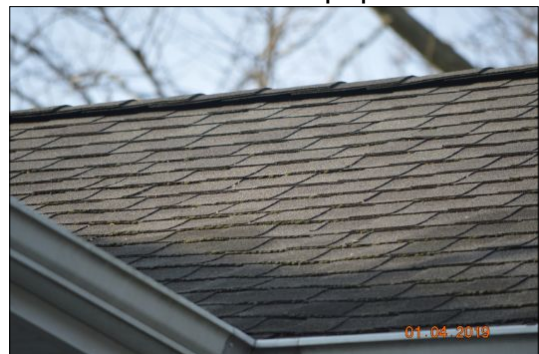
Moss growth - rear roof
