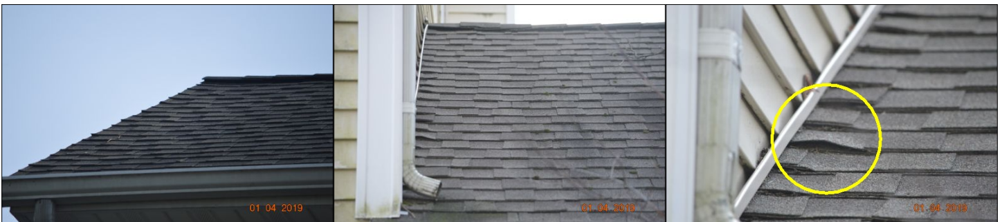
Nail pop - rear roof
