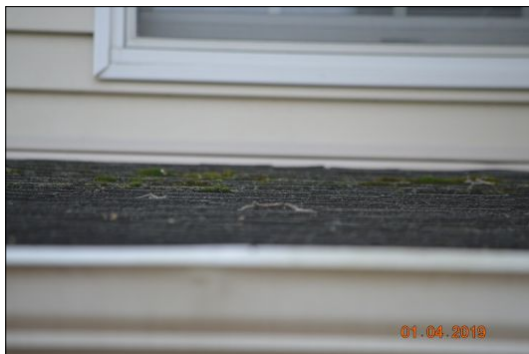
Moss growth - rear roof
