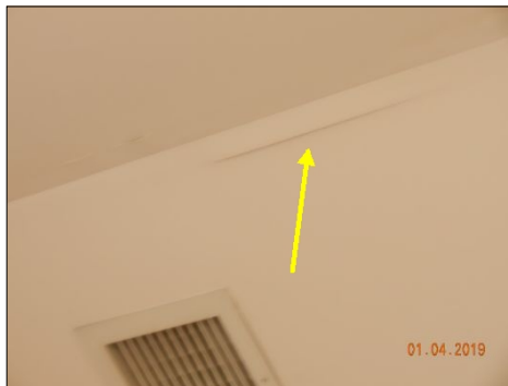
Peeling joint tape
