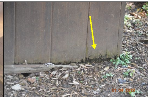
Missing and damaged trim on front porch
