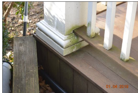
Loose and damaged railings
